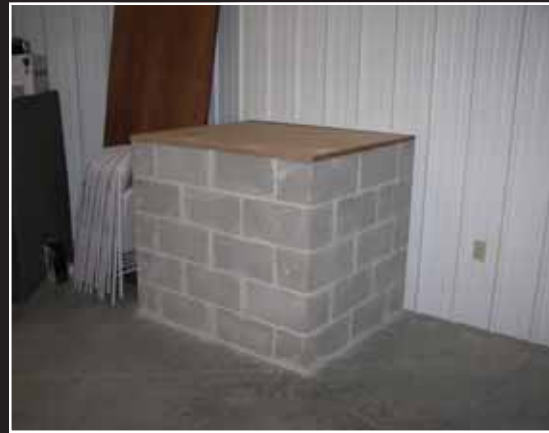
On the non-public side of the stage, the concrete block bunkers housing the sub-cabinets are filled with sand.
